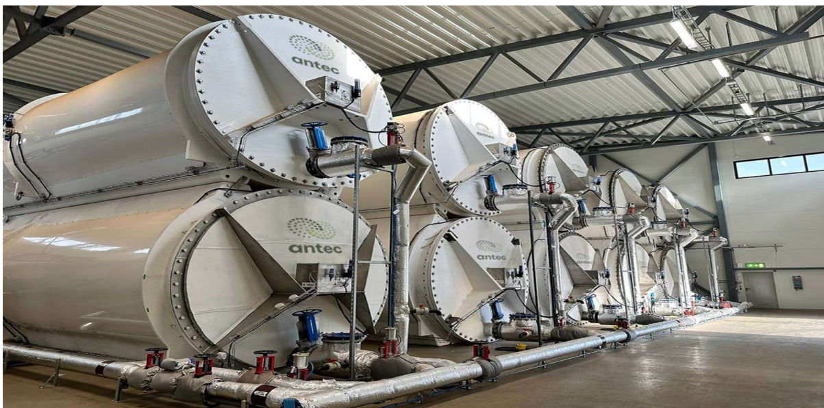
Plate 2: Typical Reactor Bank
